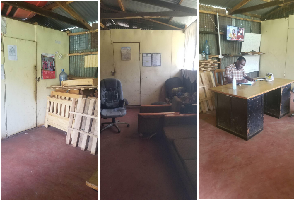
Fig 3. The current Fire Station Administration area which also serves as day room,dining room,storage unit etc.
